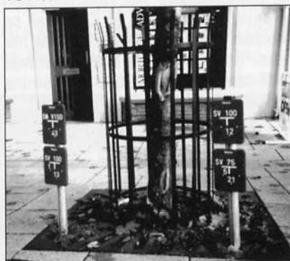
A rash of blue water valve markers
