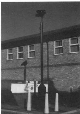
Security camera already operational in Water Lane car park
